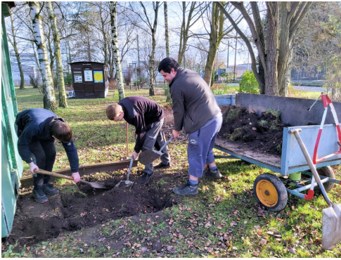
Robert Smith, Josh Sharp and Mark Boulton excavated an area at one end of the green tram, ready to take sets and rails.
