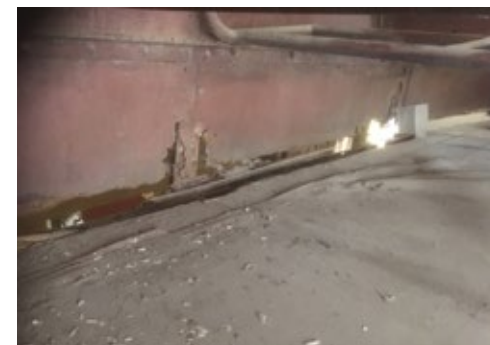
Above: “As found” – the upper deck near-side lino-covered floor and some well-rotted body structure. Stripping the lino off revealed around 12” of the floor timber had rotted away. The seat rail (top of photograph) arguably held this part of the body together.
