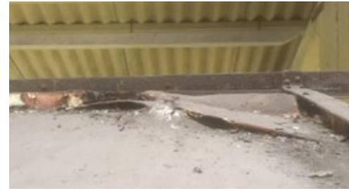
Above: The off-side of the rear roof dome: the vertical handrail stanchion at the top of the stairs has punched through the aluminium causing additional splitting. Probably, a weakened dome from a rear-end accident, combined with a violent dewatering and subsequent body movement caused all this.
