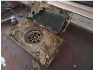
View on the roof of one of the corroded vent units after part removal (DS)
