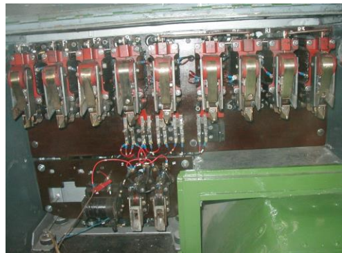
End-result: the refurbished sets of contactors now installed in the cab of 105, including the smaller ex-Sandtoft shunt field panel below
