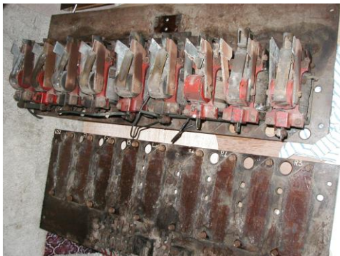
Starting-point: the salvaged contactor panels in the process of being stripped down and rebuilt Photos: Bruce Lake
