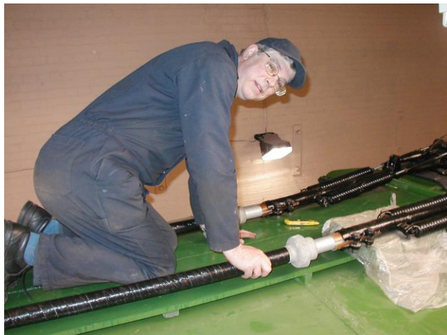
Bruce in the process of re-threading the boom cables and making the necessary connections on the roof.
