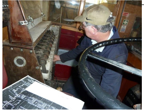
At the other end of the process, Bruce looking into the contactor box and referring to the circuit diagrams (24 April)
