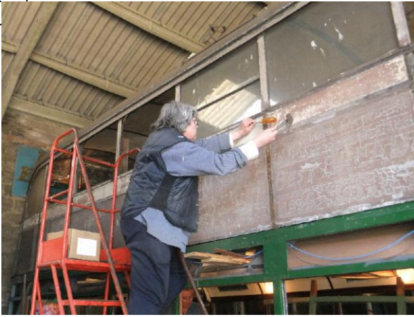
Steve Collins removes 367's upper deck beading and panels Photos: Andy Thornton
