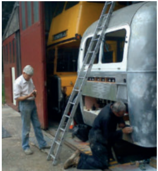
Work underway on the contactor cabinet, which is located under the back seat: a design feature to allow maximum space for seating at the front of the vehicle. Photos: Mike Johnson
