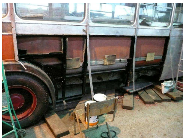
Above: Renovation of the underlying framework whilst the lower side panels are removed
