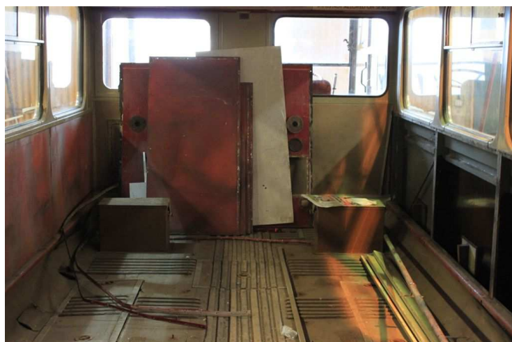
4 March 2013: lower deck interior seats removed and panels being taken off Photo: Bob Ashton
