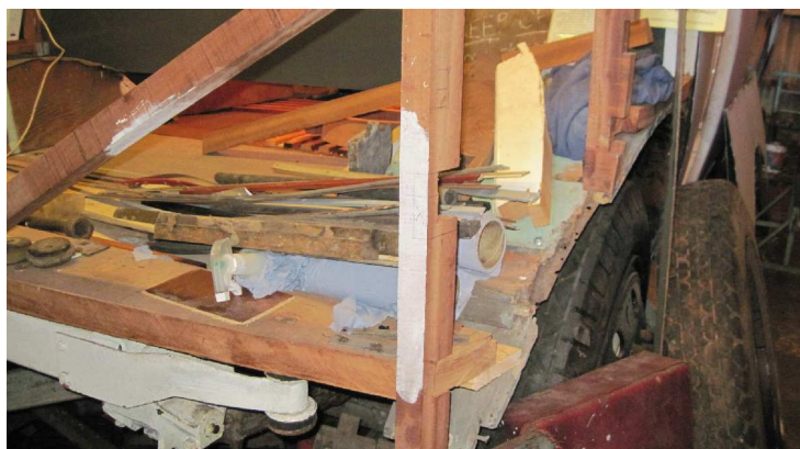
New timber taking shape to form the structure of 562's cab front and wheel arch Photo: John Crossley
