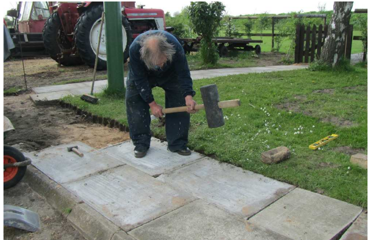
Improvements to paved areas have been happening all around the Museum ... thanks to John Whipham, seen here wielding the mallet
