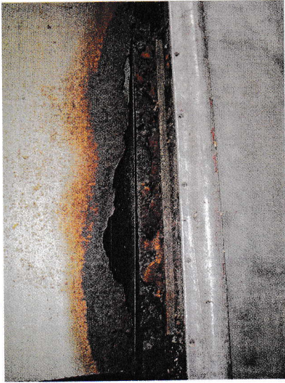
One of several severely corroded upper deck stress panels that had to be replaced Photo: John Crossley
