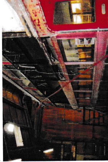
New stress panels in place on the upper deck near side Photo: John Crossley
