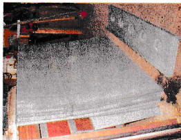
New stress panels for below the lower-deck windows (left) and the cant rail (right)
