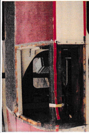
Close-up of the repair to the "porch" with outer panel and rotten wood removed, awaiting fitting new wood and new panel Photo: Jim Sambrooks
