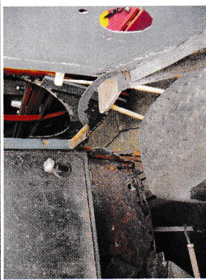
Where 758's nearside front wheel arch and cab floor isn't (but should be)!
